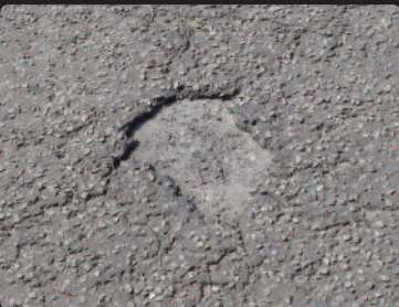
➤ A typical pothole
